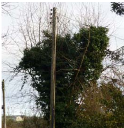
Tree interfering with overhead lines
