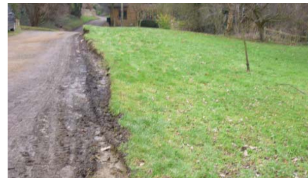
Soft edges are prone to erosion
