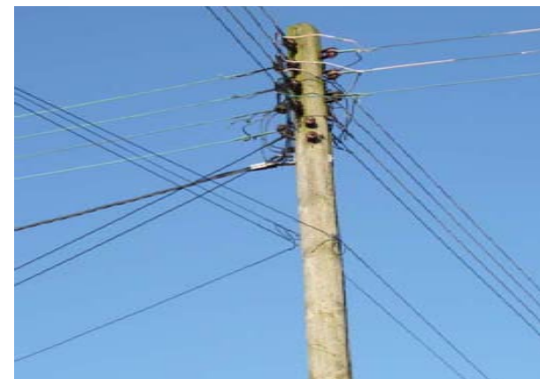
Visual impact of overhead wires
