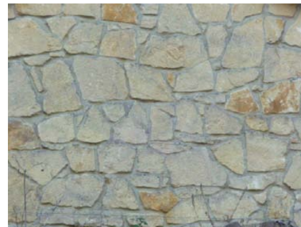
'Crazy paving' style stonework. Non local stone laid in non load bearing manner
