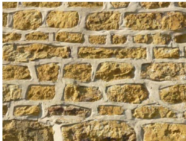
Ribbon or tuck pointing should be avoided as it causes the ironstone to deteriorate
