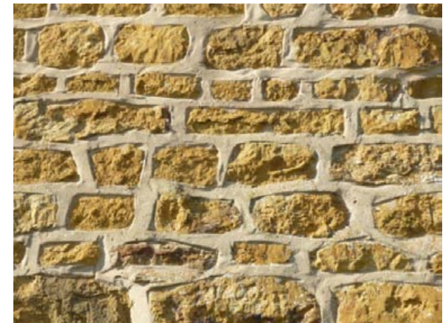
Proud pointing with cementaceous mortar can accelerate the erosion of the soft stone
